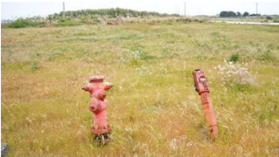
Figure 2-29: Open Storage Vegetated Areas and Fire Protection Utilities
