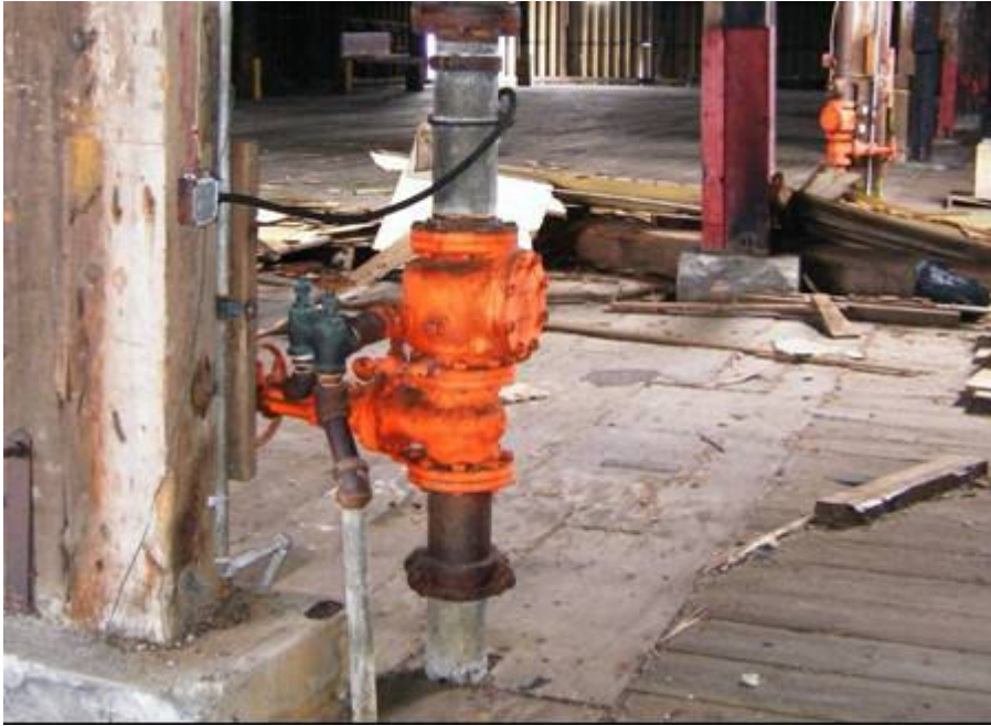
Figure 2-8: Warehouse 14 Fire Sprinkler Shut-off and Check Valve
