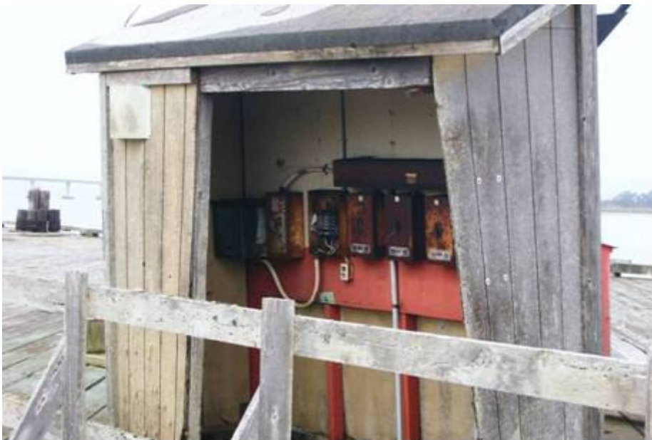
Figure 2-21: Berth 1 On-Dock Electric Switch Box
