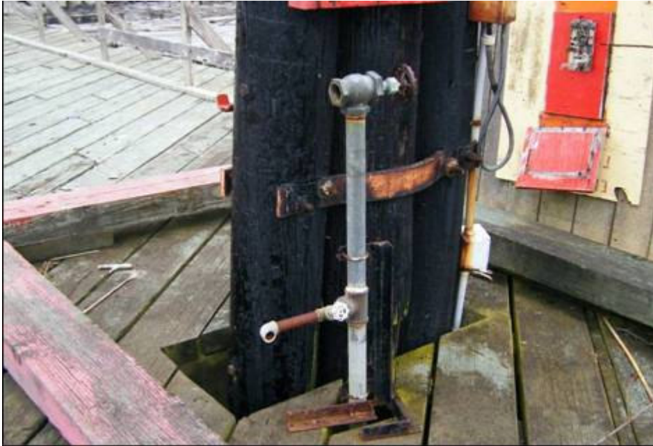
Figure 2-22: Berth 1 On-Dock Fire Control Pressurized Stand Pipe
