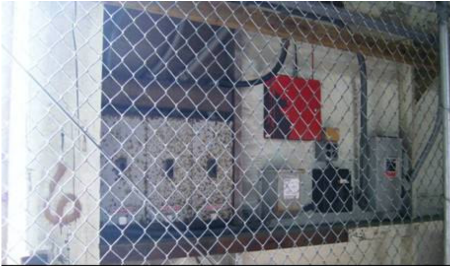
Figure 2-13: Electrical Junction Box
