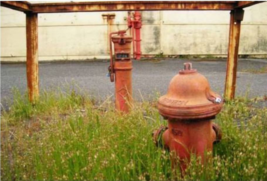
Figure 2-12: Warehouse 3 External Fire Protection and Fire Main Control
